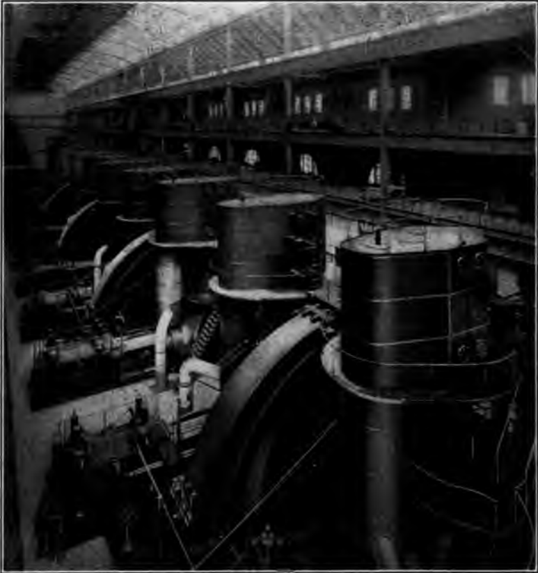
FIG. 17.—Manhattan type duplex cross-compound engine. Subway Power House, New York.
